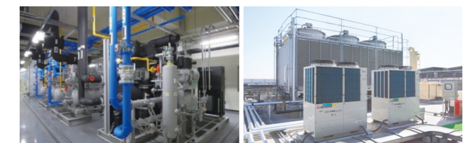
Hybrid refrigerant equipment
